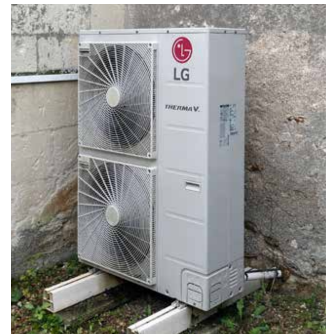
Example of a heat pump installation.
