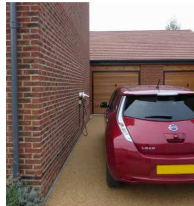
Home electric vehicle charging
